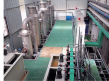
Zero-discharge wastewater equipment in the Wuxi Rite (Wuxi factory)
